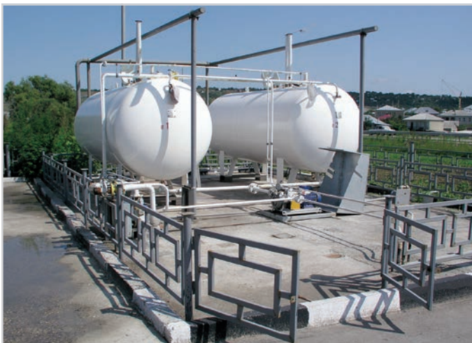
Aboveground autogas installation using one autogas series pump with two tanks.
