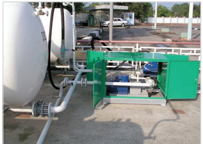
Aboveground autogas installation using one autogas series pump with three tanks.
